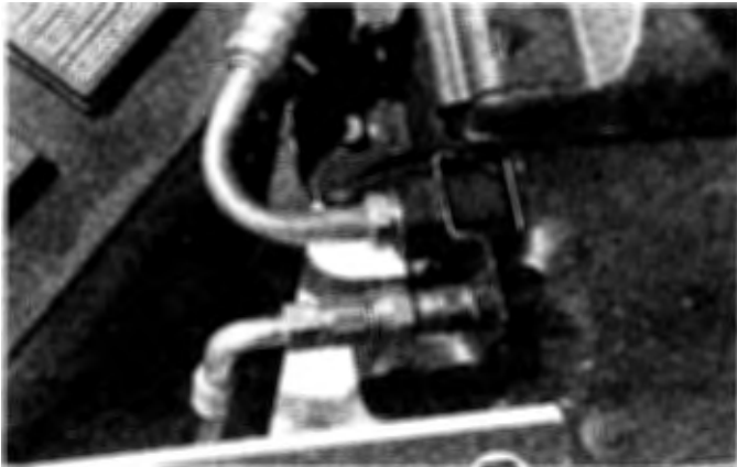
15.5c On four-cylinder and V6 models, the refrigerant line connections are located next to the battery
