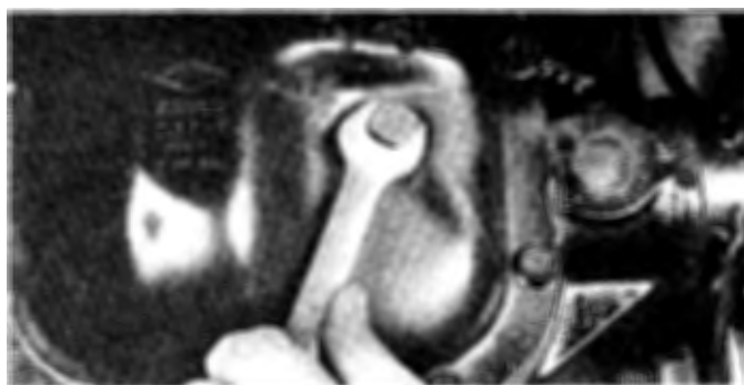
17.2 Use the correct size open-end wrench to remove the differential check/fill plug
