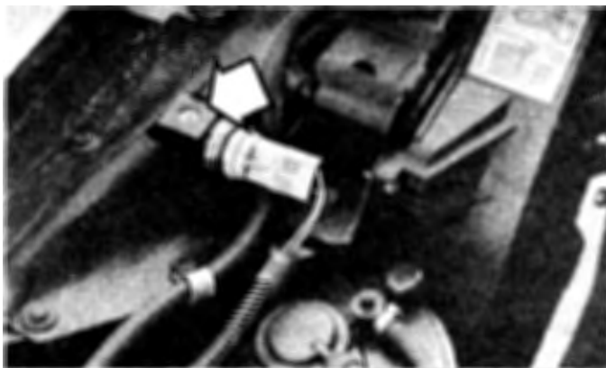
12.7a On four-cylinder and V6 models, the sight glass is adjacent to the radiator cap (arrow)
