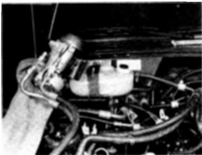
5.12 Unbolt the air conditioning compressor and set it out of the way
